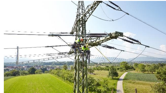
Electricity distribution infrastructure
