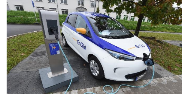
E-mobility charging infrastructure
