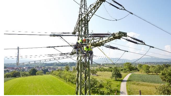
Electricity distribution infrastructure
